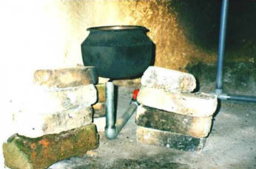
Figure 15. Biogas is brought to the kitchen using PVC connections, due to its corrosive action. Only the last tube is a iron galvanized pipe. A biogas plant can produce enough fuel to fulfill the requirements of a rural family.
