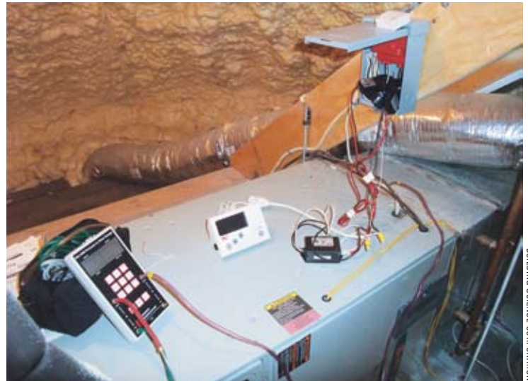
Measurement procedure, showing digital manometer (Energy Conservatory DG-700) and power meter (The Energy Detective). TrueFlow airflow measurement plate is inside filter slot.
