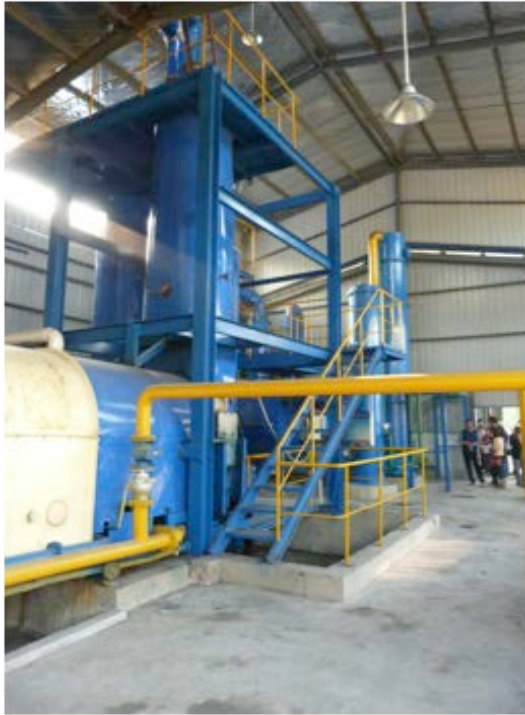
Visit to Nintan Biochar Demonstration Plant in Nanjing, affiliated with biochar center of Nanjing Agricultural University. Rotary kiln pyrolyser working.
